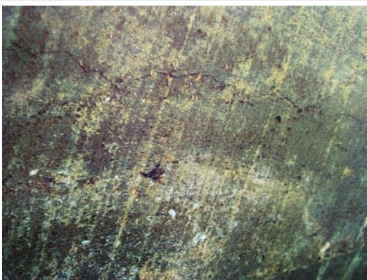
Figure 5: Yield line pattern noticed on slab.
