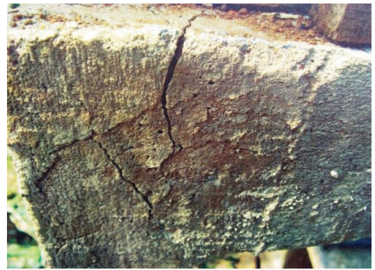
Figure 6: Cracks noticed on the beam/column joint.
